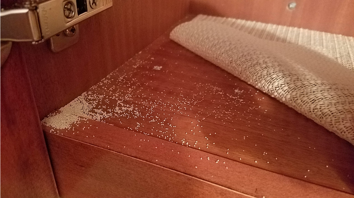
David inspected the inside of the cabinets and the tops of the cabinets. The matter was prevalent in all of the cabinets.
